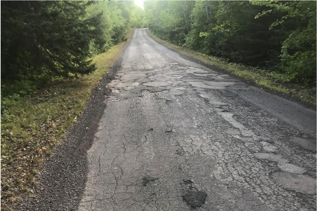
Deteriorated Pavement (Typical)
