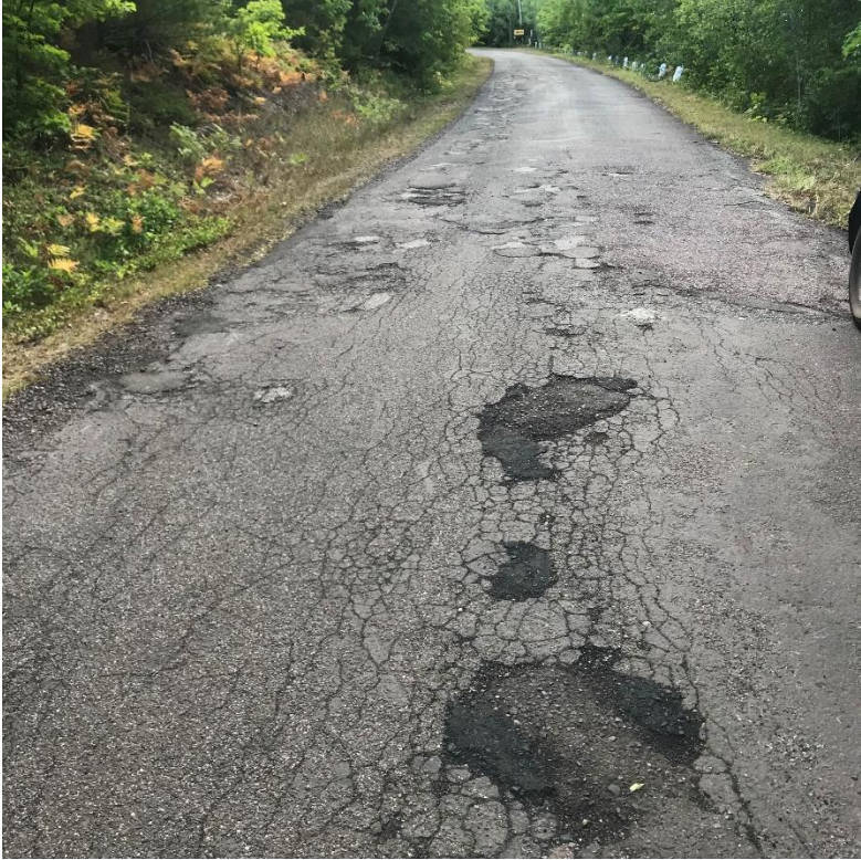
Deteriorated Pavement (Typical)
