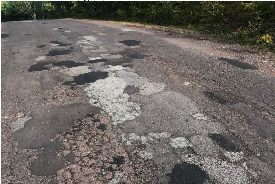
Deteriorated Pavement (Typical)
