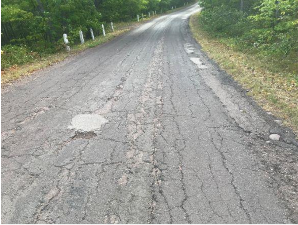
Deteriorated Pavement (Typical)
