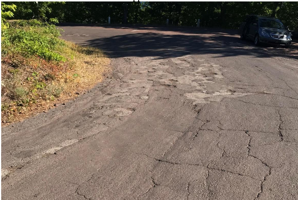
Deteriorated pavement at eastern look-out approach (Typical)
